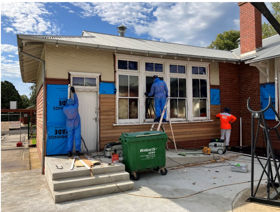
Above and Below – Refurbishment of the external surface of the HLC is also occurring and will be completed by Open Day. Thanks to our former and current HLC Managers for initiating this project and seeing it come to fruition!
